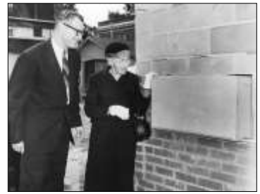
December 22, 1957 Rev. Turner and Mrs. Georgia Newsom at the laying of the Education Building's construction.
